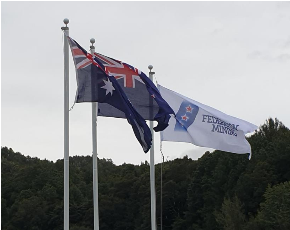
During the month the team installed a series of flag poles for the New Zealand, Australian and Federation flags
